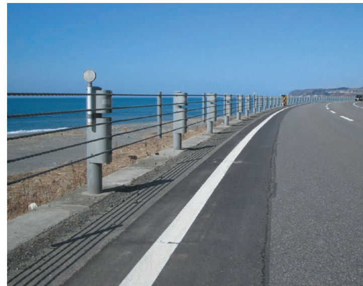
"Guard Cables" use the elasticity of wire ropes to absorb energy during a vehicle collision. They have the highest transparency and can make the road appear wider.
