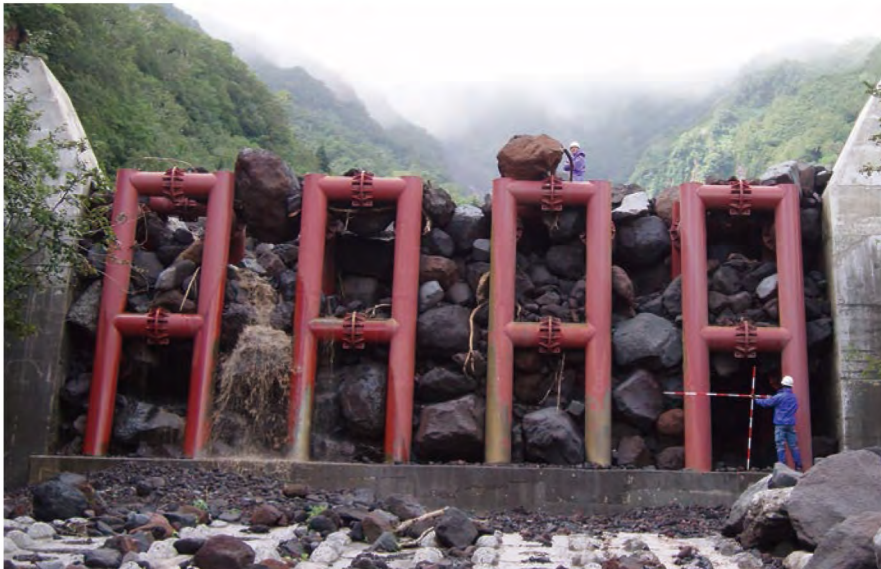
Steel Slit Dam Type B
